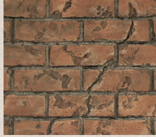
Fire Cracked Brick
