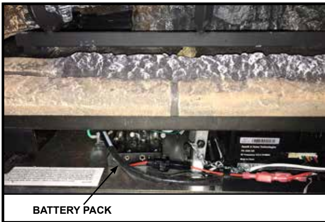
Figure 6.3 Battery Pack Installed
