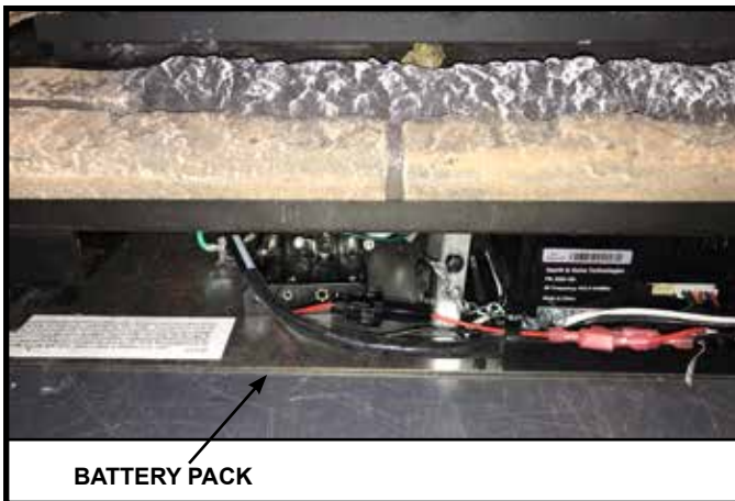
Figure 6.3 Battery Pack Installed
